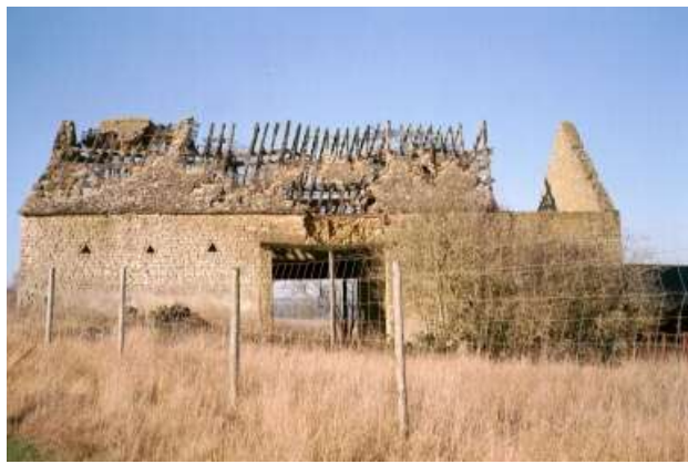
Top Barn at Walcot, near Charlbury - derelict in 2003
