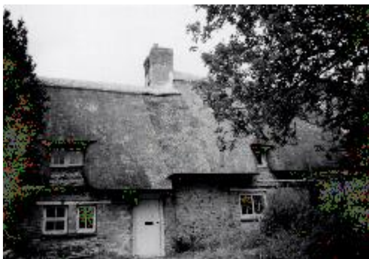
Wayside from the south, shortly after repairs to the section around chimneys, June 1999. Early 14 th C hall to west (left), mid-14 th C hall to east of inserted chimney, later stone walls and attic chambers
