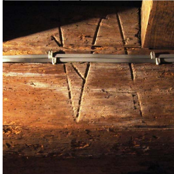
Above: an example of Baltic timber marks recorded by OBR members in Abingdon Long Gallery. This set is on a softwood transverse beam inserted as an 18 th century alteration to the ground floor.
