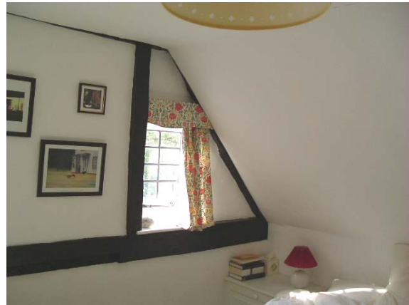
Unaltered end of same truss
